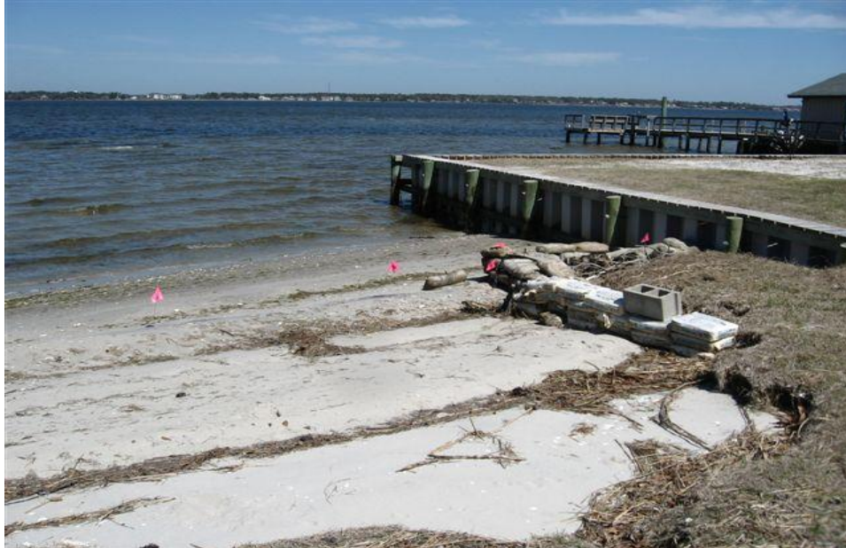
View of Mr. Hollings bulkhead adjacent to the Caldwell's eroded shoreline in the spring of 2013. The Caldwell's have placed sandbags next to Mr. Holling's property to temporarily prevent further erosion. Photo credit: R. Gittman
