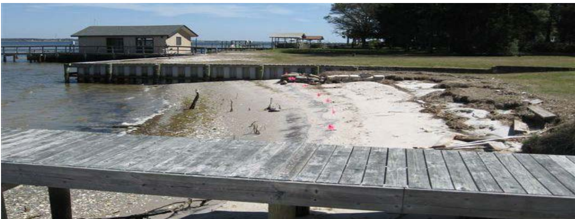
The current condition of the Caldwell's shoreline. Mr. Holling's property is shown in the background. Photo credit: R. Gittman
