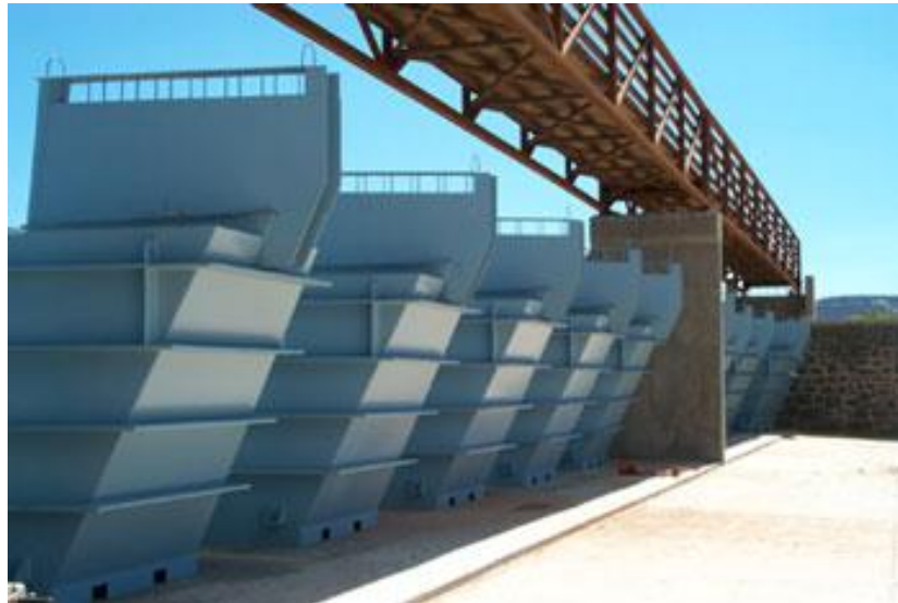
Fusegates Installed at the Black Rock Dam
